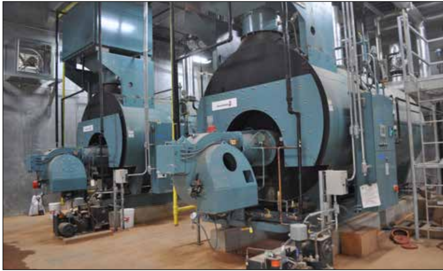
Two Cleaver Brooks 500-hp boilers supply steam for pelleting operations.
