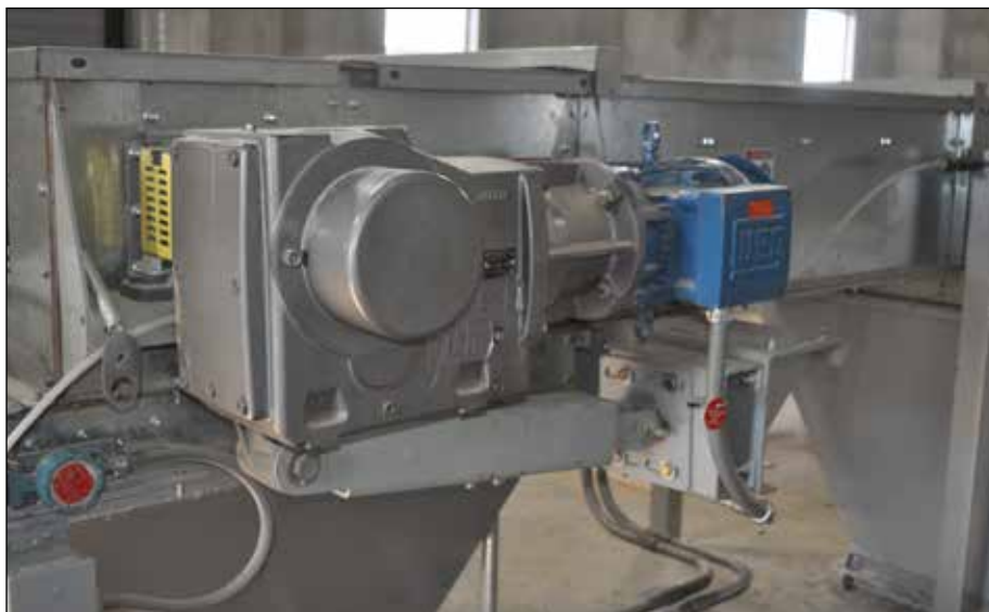
Nord direct drive utilized on most of the equipment in the mill.
